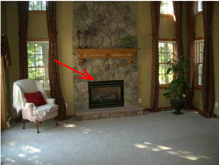
Family Room---Gas fire place, direct vent
