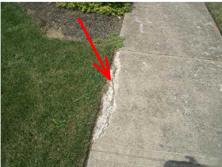
Walkway---concrete, cracked and deteriorating also trip hazard
