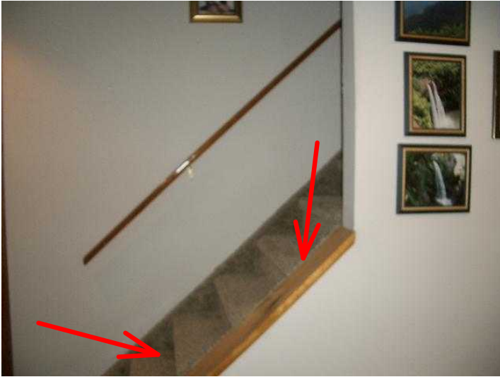
Basement Stairs---install safety rail
