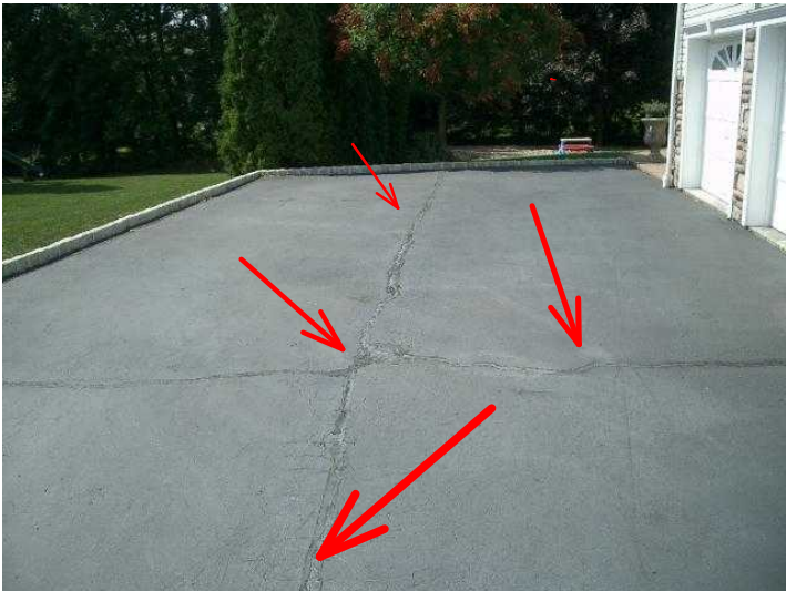
Driveway---cracked, recommend repair or replacement
