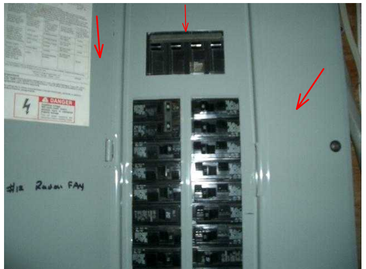
Electric---Main Panel in basement---200 amps estimate
