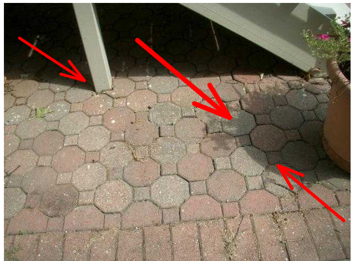
Rear Stairs---supports appear to be in direct contact with soil, also depression in pavers.
