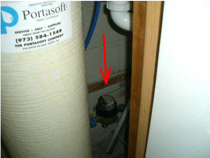
Water Meter -----in closet
