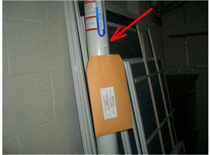
Radon System---in basement
